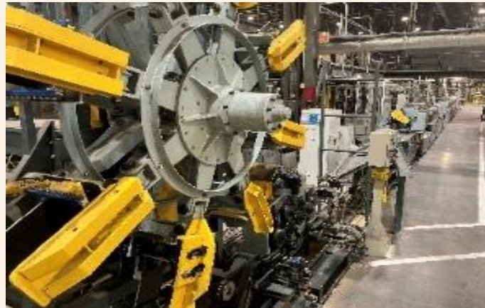
Equipment inside the plant
