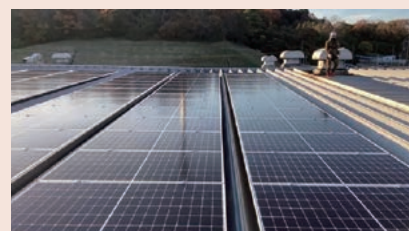
Solar power panels (Kobe Plant)
