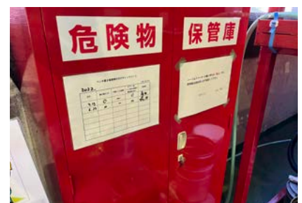
Management of chemical substances
