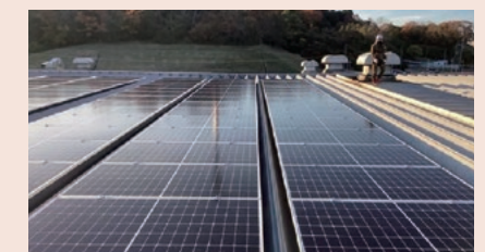
Solar power panels (Kobe Plant)
